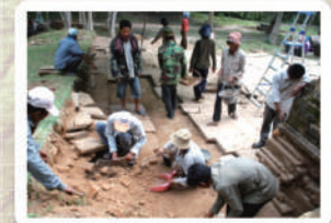
The clearance work on the terrace, cooperated with villager and local worker of SCP (SCP)
