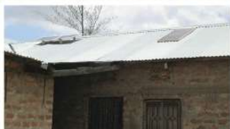
The solar panels on the roof
